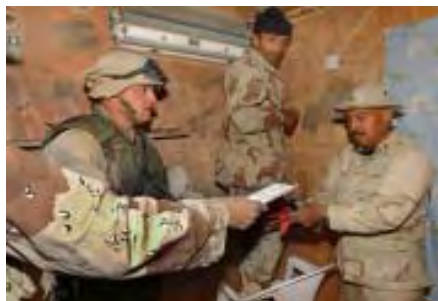
EO3 Michael Martin, left consults with SW2 Jesus Cepeda, far right during an air conditioner installation in the ISF camp. ISF troops interested in learning about the equipment helped install it.
