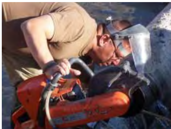
Ramon uses a hand-held concrete saw to cut into the water main to replace the damaged section.
