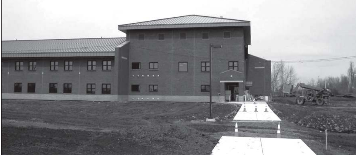
The Divarty Barracks are being constructed at Fort Drum to house single Soldiers.
