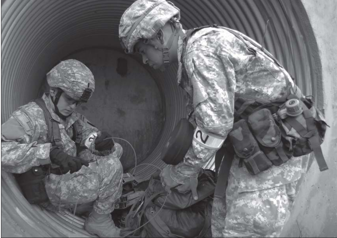
A team from the 66th Engineer Company prepares their charge during the steel-cutting charge evaluation.
