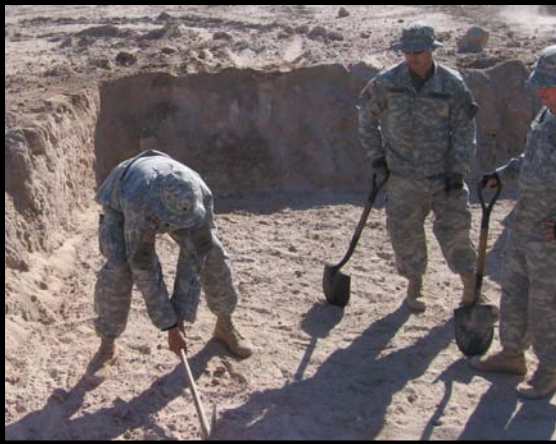
Top Left: Breaking ground, Pvt. 2 Michael N. Ripp from 1st Platoon, Company C, 40th Engineer Battalion, of TF Conqueror uses the Bobcat to dig the hole for the evaporation tank. Bottom Left: PFC Billy A. Daffron and Sgt. Bryan J. Osborne of Company C, 40th Engineer Battalion, of TF Conqueror, watch as Spec. Kenneth J. Stroede uses a pick mattock to break through a hard spot while trying to create a level base for the evaporation tank for the 2nd Brigade Combat Team's new washrack facility. Right: The 2nd Brigade Combat Team's improvised washrack was completed January 8th, 2006, at Camp Buehring, Kuwait.
