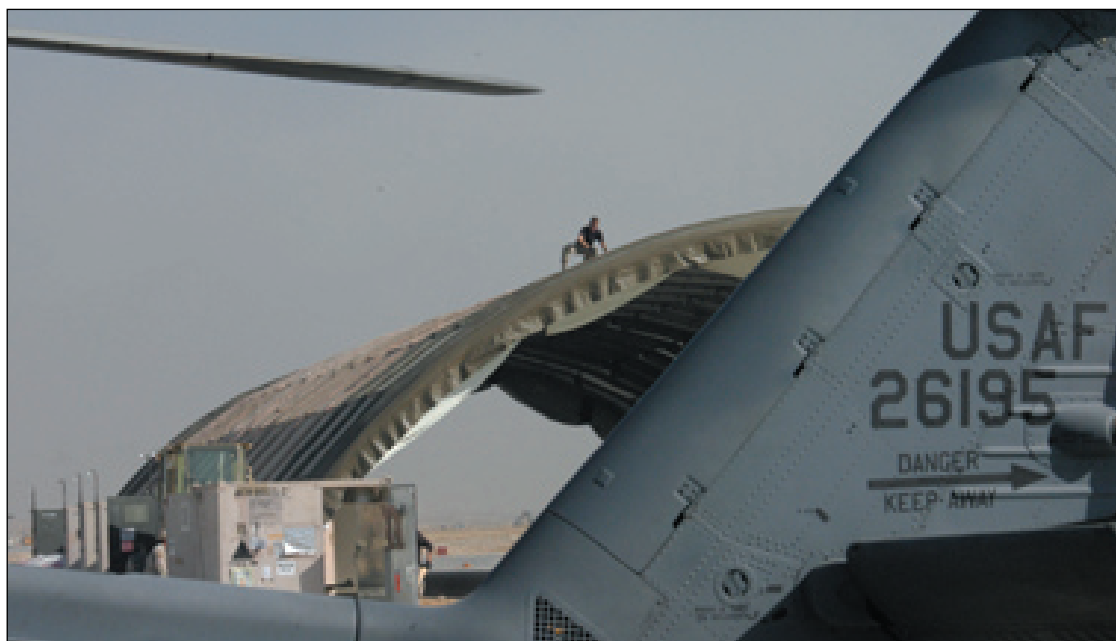
Senior Airman Brad Hellberg puts the finishing touches on the Air Force's largest-ever deployable aircraft hangar at Bagram Airfield. The hangar is intended to simultaneously house up to three of the 455th Air Expeditionary Wing's combat search and rescue HH-60 Pave Hawk helicopters. A nine-person team erects and tears down similar structures throughout the U.S. Central Command area of responsibility.
