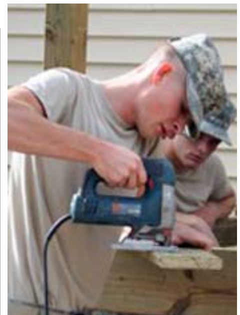
Specialists Nathan Johnson and Corey Merkel construct a deck at a home in Ridgeway, Iowa. Work there also included drywall and siding installation, as well help with landscaping.
