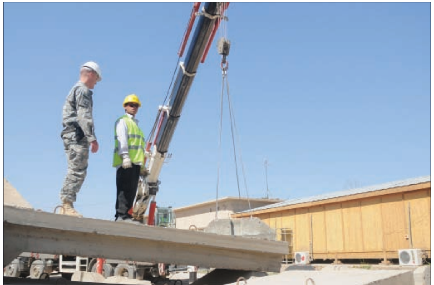
Sgt. Robert Bernstorf, the barrier protection sergeant with the Regimental Fires Squadron, 278th Armored Cavalry Regiment, 13th Sustainment Command (Expeditionary) and a Kingston, Tenn., native, and a local national worker watch as a crane moves a T-wall closer to the building to provide barrier protection, April 15 at Contingency Operating Base, Marez, Iraq.
