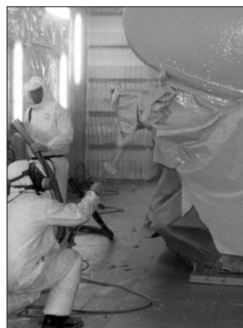
Workers apply a TankSkin protective coating on a fuel tanker, which can deflect bullets and seal up to .50-caliber-sized holes.
