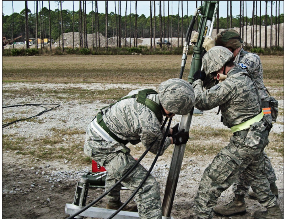
124th Civil Engineer Squadron power production specialists construct a mobile aircraft arresting system during their weeklong Silver Flag exercise in February at Tyndall Air Force Base, Fla. (Photo courtesy of 124 CES)
