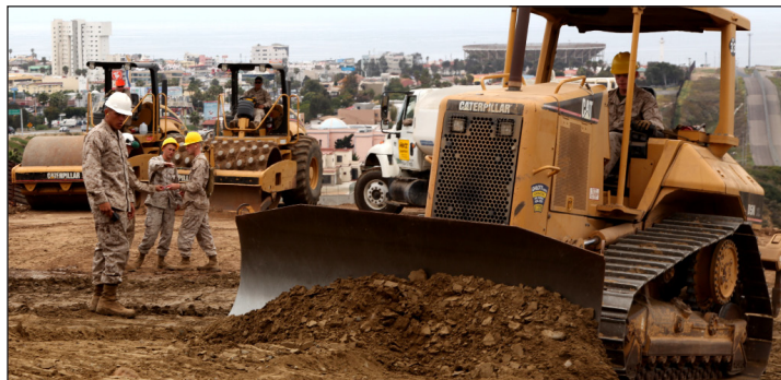
Marines with 7th Engineer Support Battalion, 1st Marine Logistics Group, build a road along the Mexican border in San Diego, April 23, in support of a Joint Task Force North operation to help improve national security and prevent foreign trespassers.
