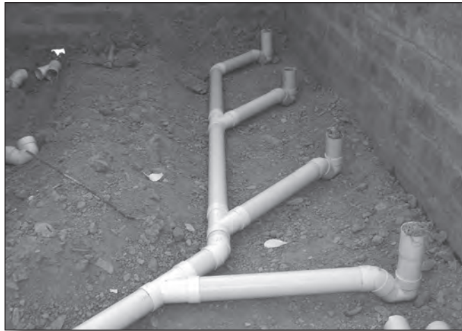
The plumbing solution included using 30 and 60 degree bends.
