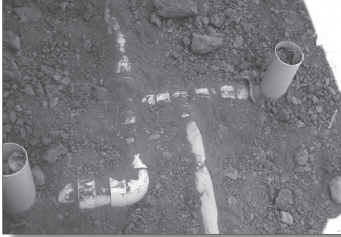
Latrine pipes with a 90 degree bend were a mistake caught by a COR.
