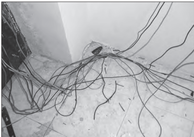
Wiring entering the building through a polyvinyl chloride pipe, wire that was too small for the load, and wire that was not double-insulated contributed to the fire.
