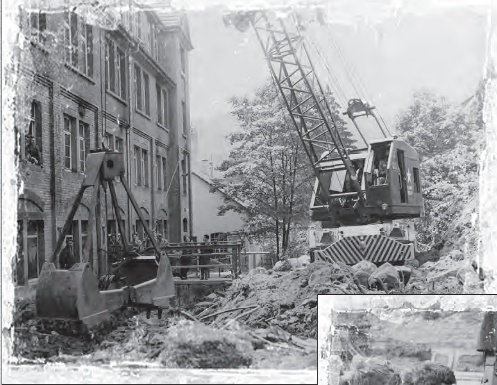
Left: A 78th Engineer Battalion crane-shovel clears debris from a Schramberg factory.
