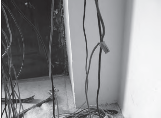
The twist-on wire connector in a hot circuit was one reason for the fire.
