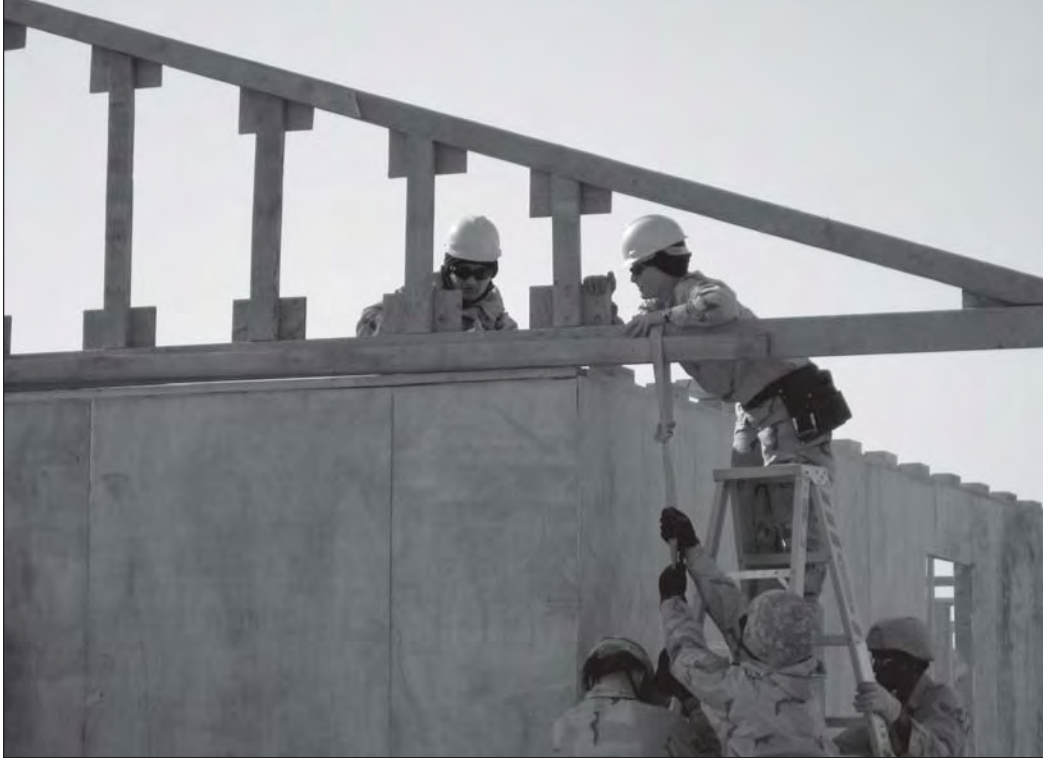
Soldiers and Airmen build a tactical operations center for the 1st Cavalry Division.
