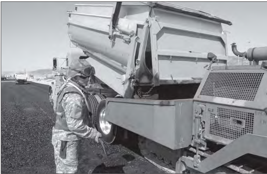
A Soldier shovels asphalt to fill in the gaps as the 770th Engineer Company repairs a section of Barstow Road at NTC.
