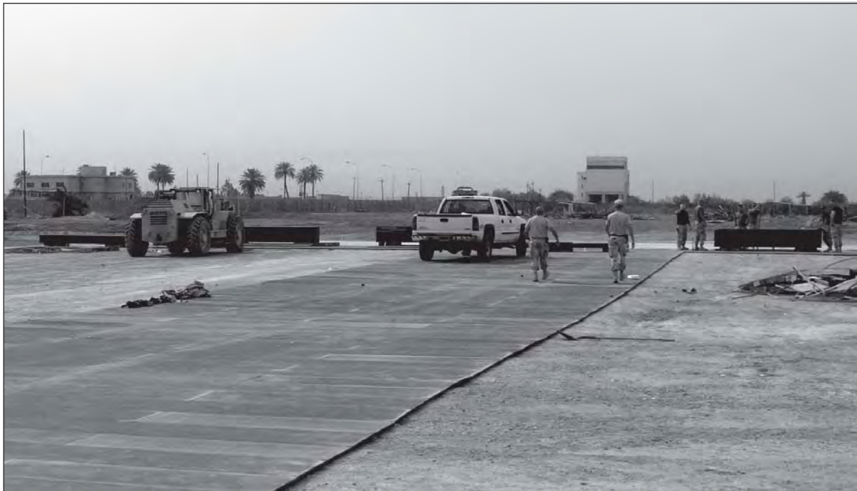
Detachment 3 Airmen construct a landing pad and taxiway for the 3d Infantry Division's Combat Aviation Brigade.
