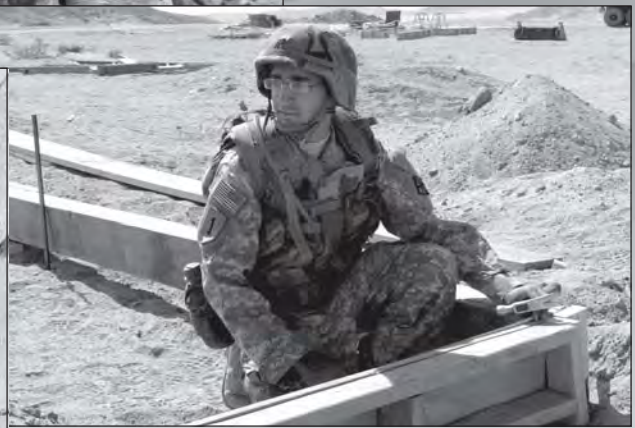
A Soldier from Company A, 854th Engineer Battalion, places forms for a building at the Medina Jabal work site.
