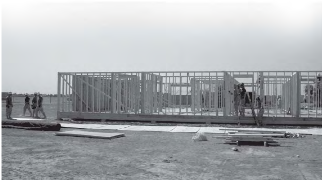
Construction on the medical treatment facility began once force protection measures were in place.
