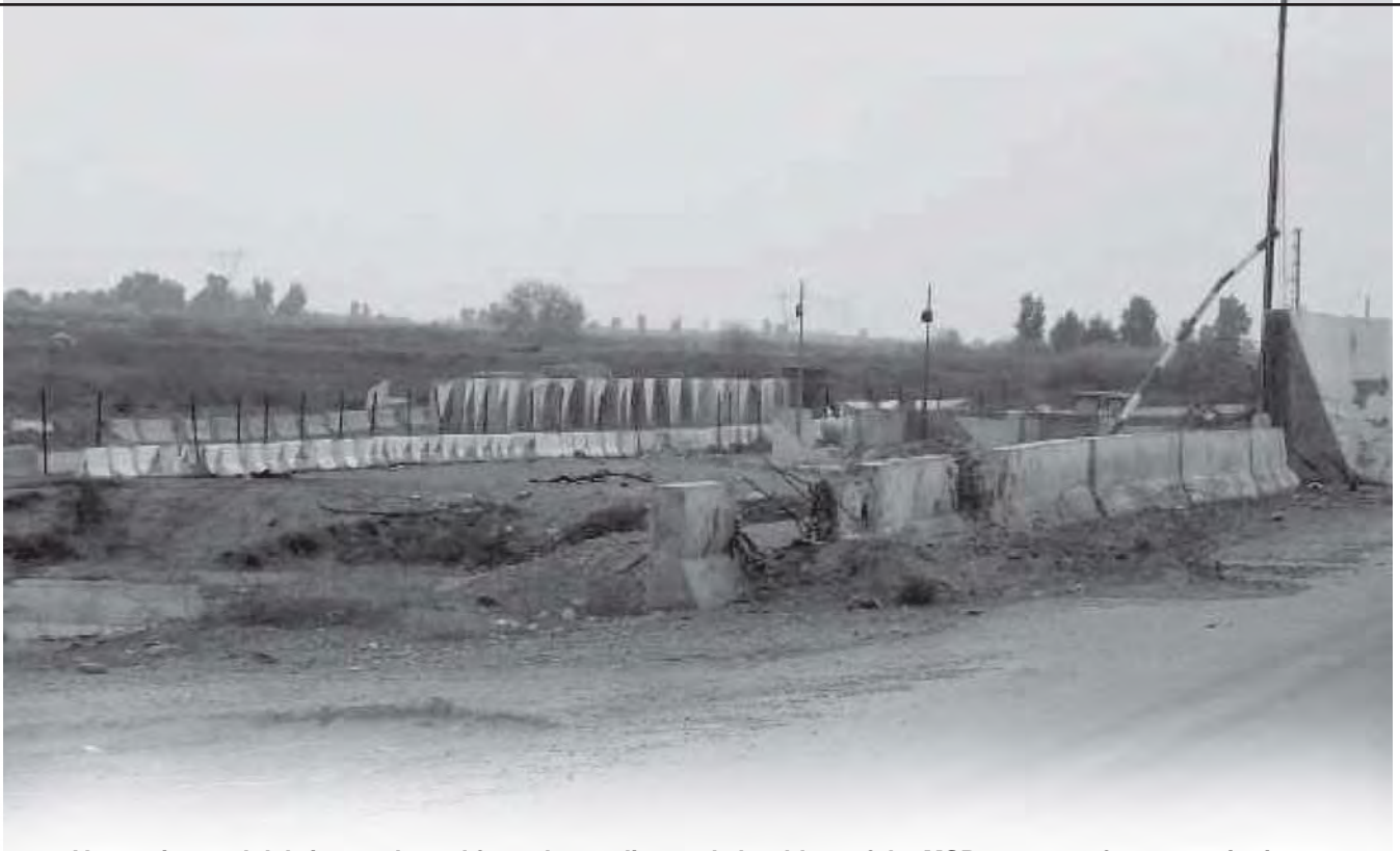
Vegetation and debris are cleared from the median and shoulders of the MSR as part of route sanitation.
