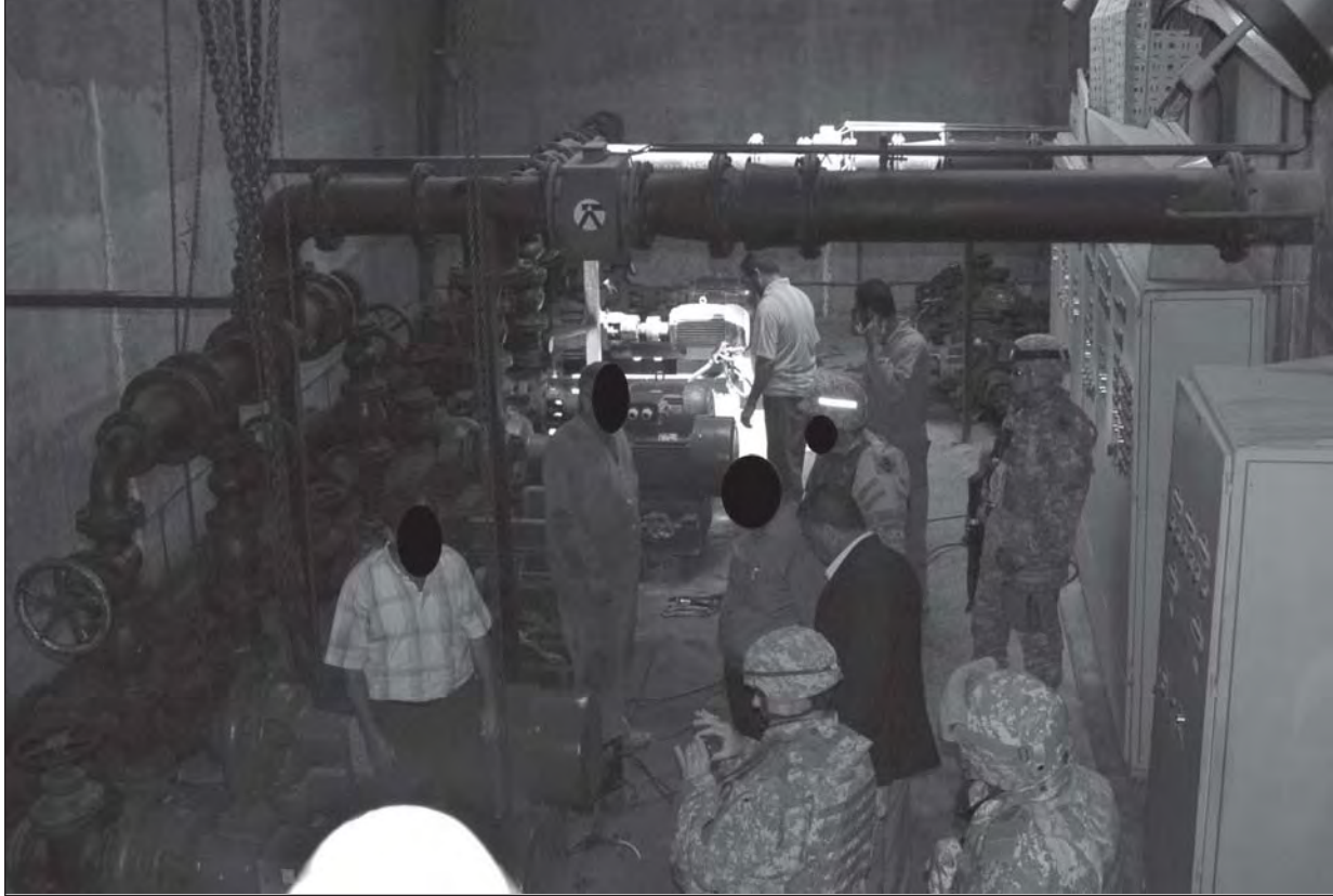
Pump station for treated water at Al Bakir
