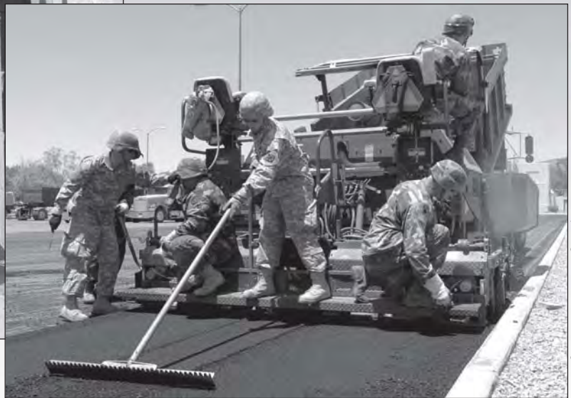
Soldiers of the 770th Engineer Company pave the parking lot of the post theater at Fort Irwin, California, as part of Operation Sand Castle.
