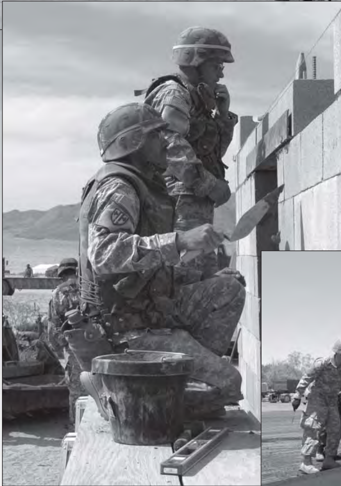
Soldiers with Company A, 458th Engineer Battalion, check for levelness while building the door frame for a building at Medina Jabal.
