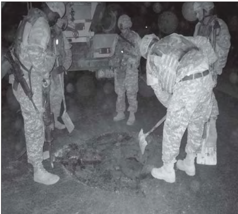
Soldiers from the 92d Engineer Battalion repair a blast hole formed by an IED detonation.
