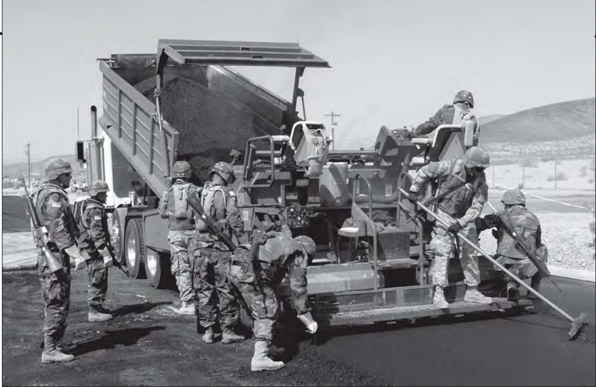
Members of the 770th Engineer Company repair a section of road at NTC in full combat gear.
