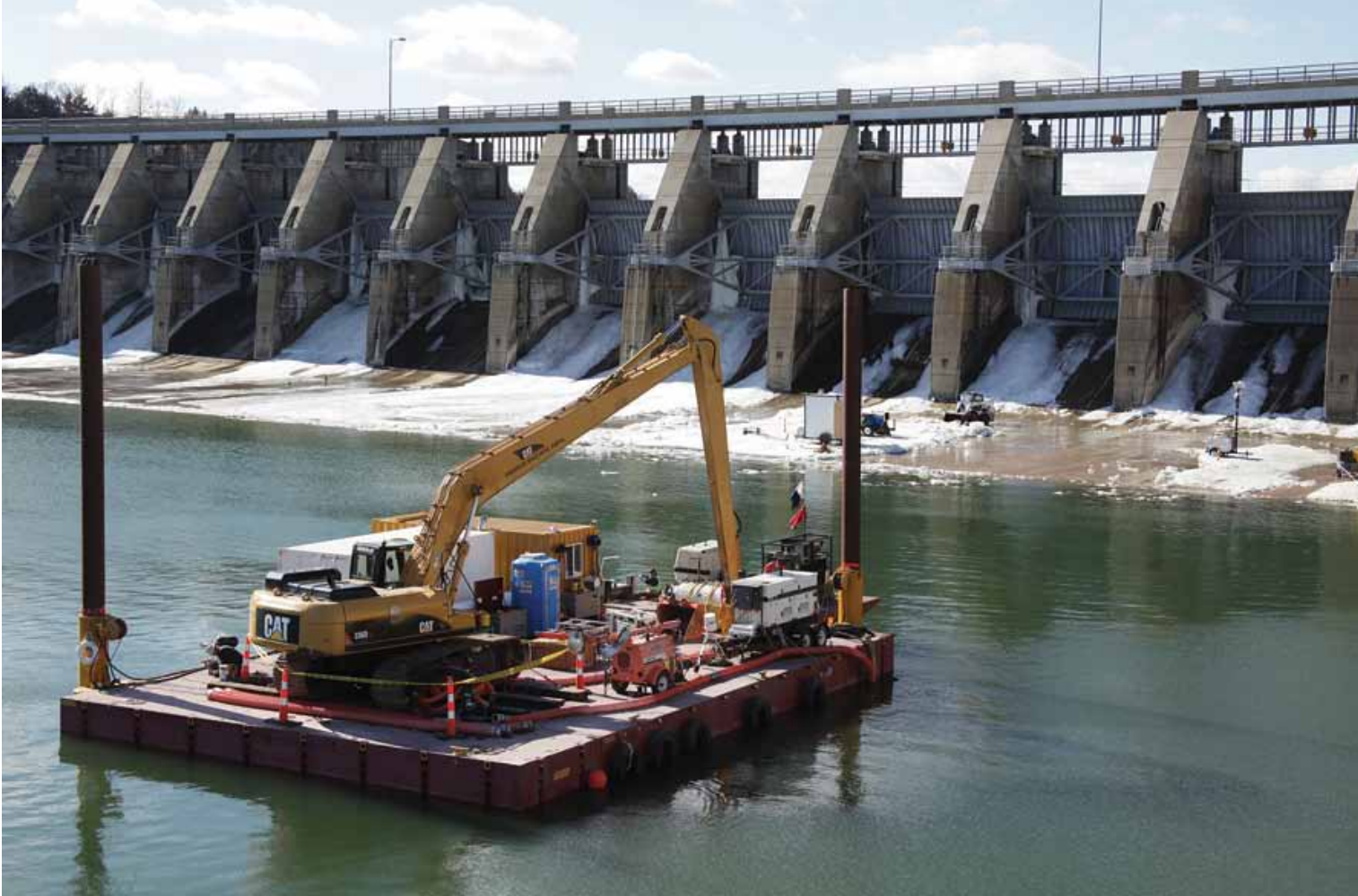
A barge station near the spillway performed tree and debris removal in the stilling basin; Lower right: crane drops riprap on the downstream river bank. All photos by Harry Weddington
