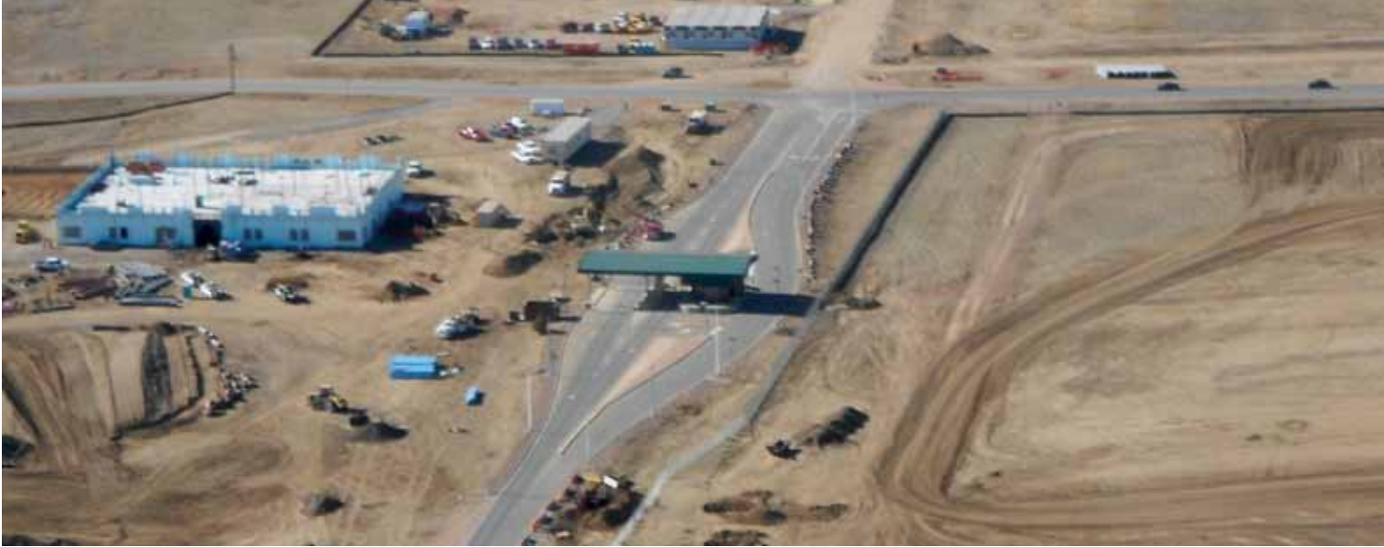
An aerial view of the construction site at Butts Army Airfield. U.S. Army Photo.
