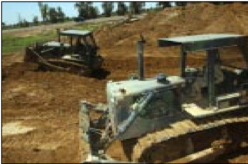
Photo by Pfc. Elizabeth Erste, 55th Signal Company (Combat Camera) Sgt. Jay Wells, and Staff Sgt. Duane Dobitz bulldoze a hole for the debris of the Ramadan 14 building, an old Baath party house located outside the city of Ad Dujayl, Iraq, that is being demolished, May 6, 2004.
