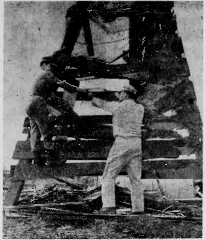
TARGET PATCHING — ASgt. Gene O. Blosky (right) and Pfc. Fred A. Marmion repair target stanchion on Molokai. The condition of the target attests to the accuracy of the MAG-13 pilots. Blosky is NCO-I-C of the six-man Marine detachment.
