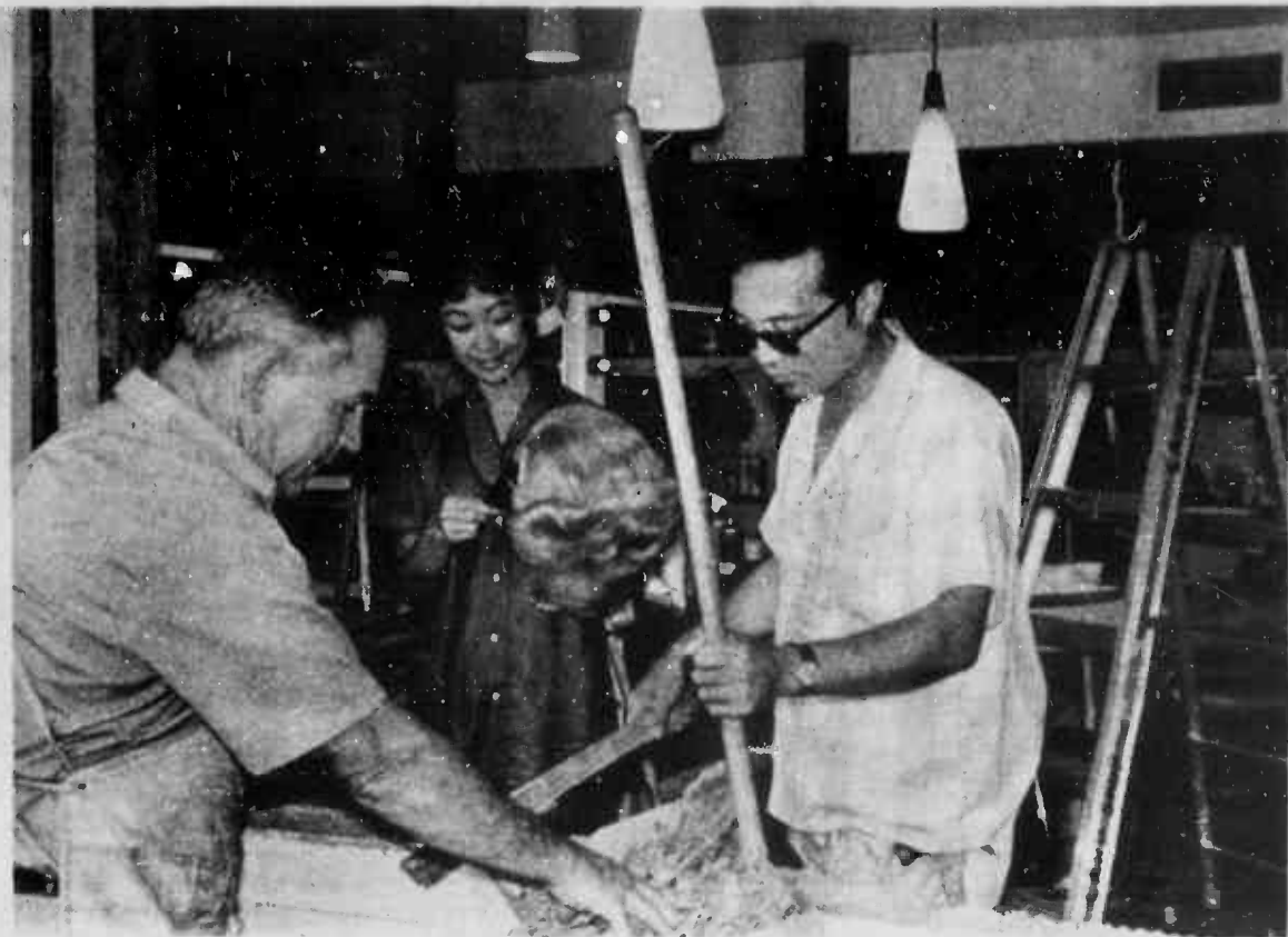
IS THIS ANY WAY TO RUN A BEAUTY PARLOR? . . . Wonders Lillian Morgan, hair stylist, as she watches Alfred Deluze (L.) and Cecil Hasegawa dispose of some wood. The Beauty Shop is being remodeled as part of a Public Works project to renovate Building 244.
