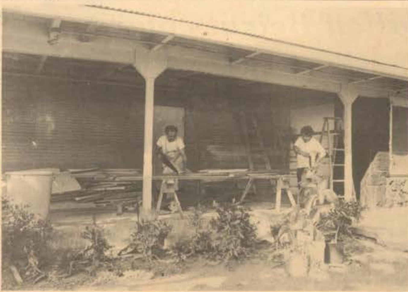
FACELIFT — Construction workers prepare to do exterior work on the 19th Puka Community Center. The renovation commenced July 17. (Photo by SSgt W.S. Saunders)
