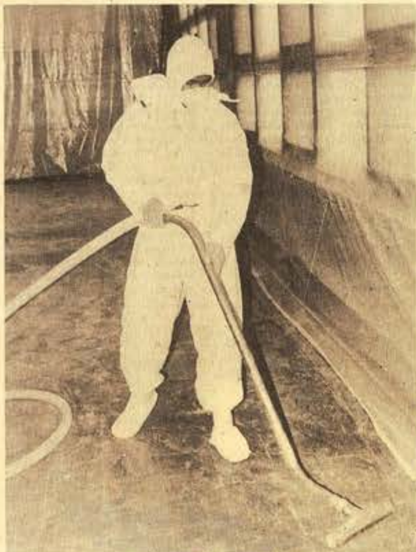
CLEANING UP — Mene Talili, Facilities Department, vacuums up asbestos fibers as part of the clean-up after an asbestos removal project in Building 220. The entire room was encased in plastic sheeting to prevent asbestos fibers from escaping and contaminating nearby areas. (Photo by Cpl Pat Lewandowski)
