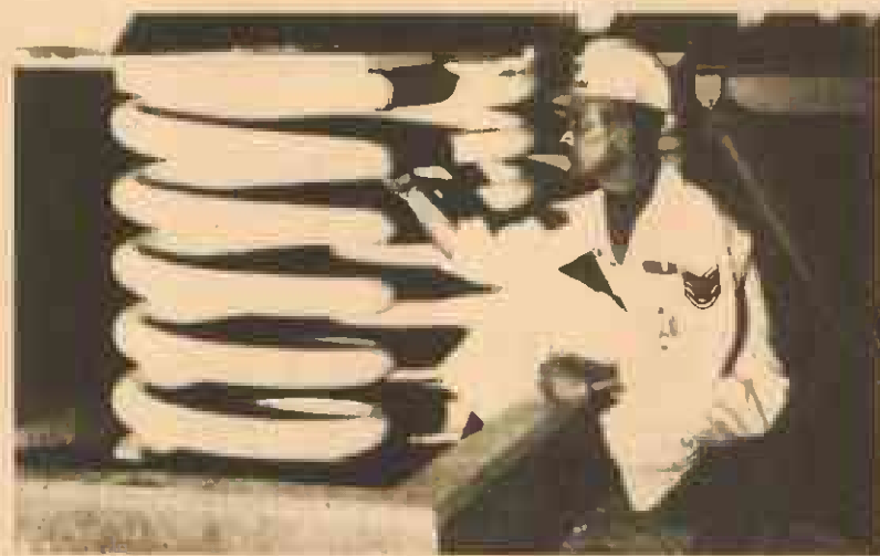
All 15 buildings in Cheyenne Mountain are placed on rows of huge steel springs, designed to protect delicate equipment. There are more than 1,300 springs, made from three-inch diameter steel rods and each weighing about 1,000 pounds.
