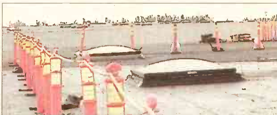
Emergency repairs, to include the replacement of two skylights, were completed Jan. 10 and 11.
