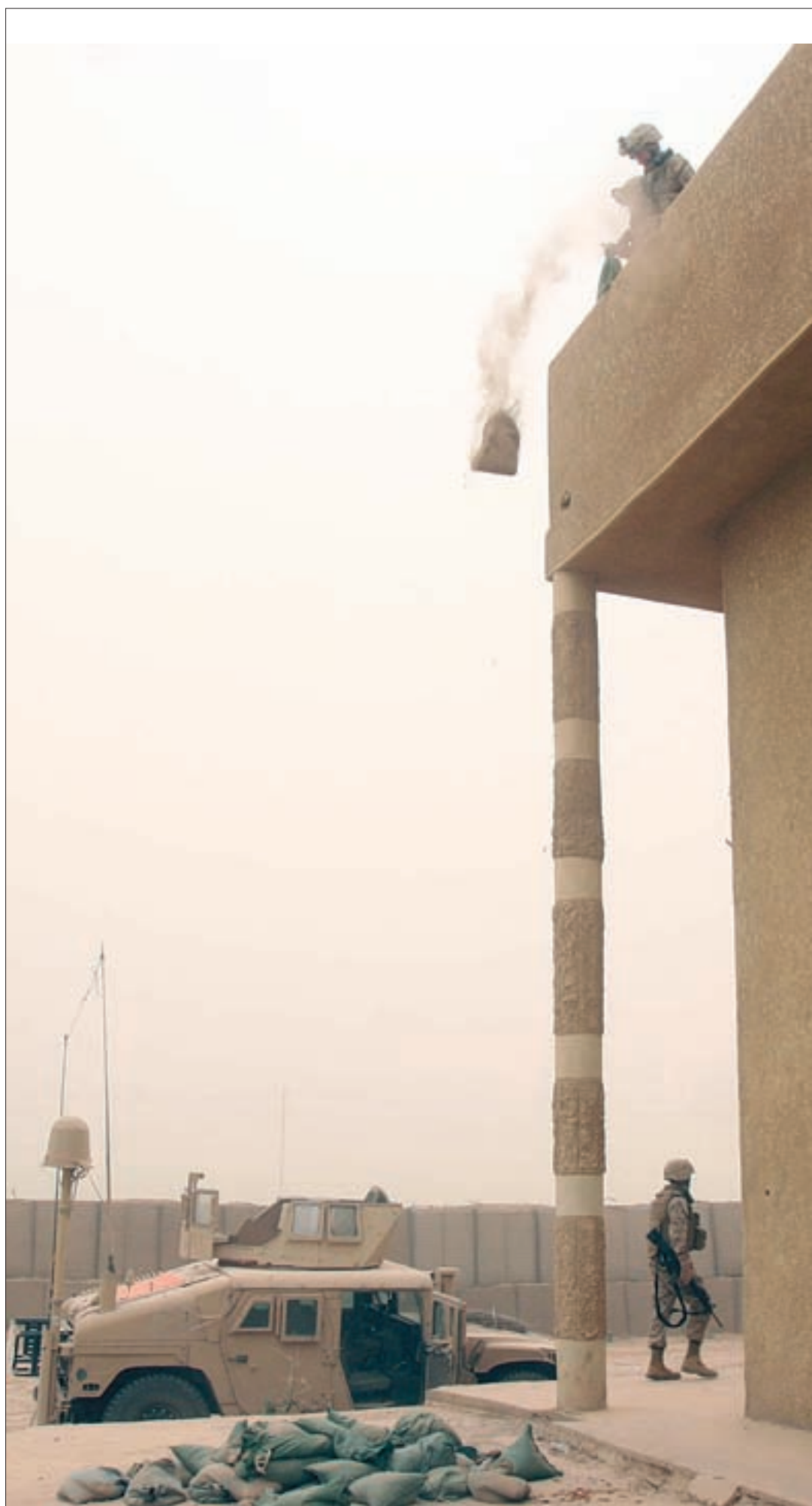
Marines with Weapons Company, 2nd Battalion, 3rd Marine Regiment, Regimental Combat Team 1, begin to toss sand bags off the roof of the Barakat house April 29, in Zaidon, Iraq. The Marines demilitarized the house where they once conducted operations alongside members of Iraqi Security Forces.
