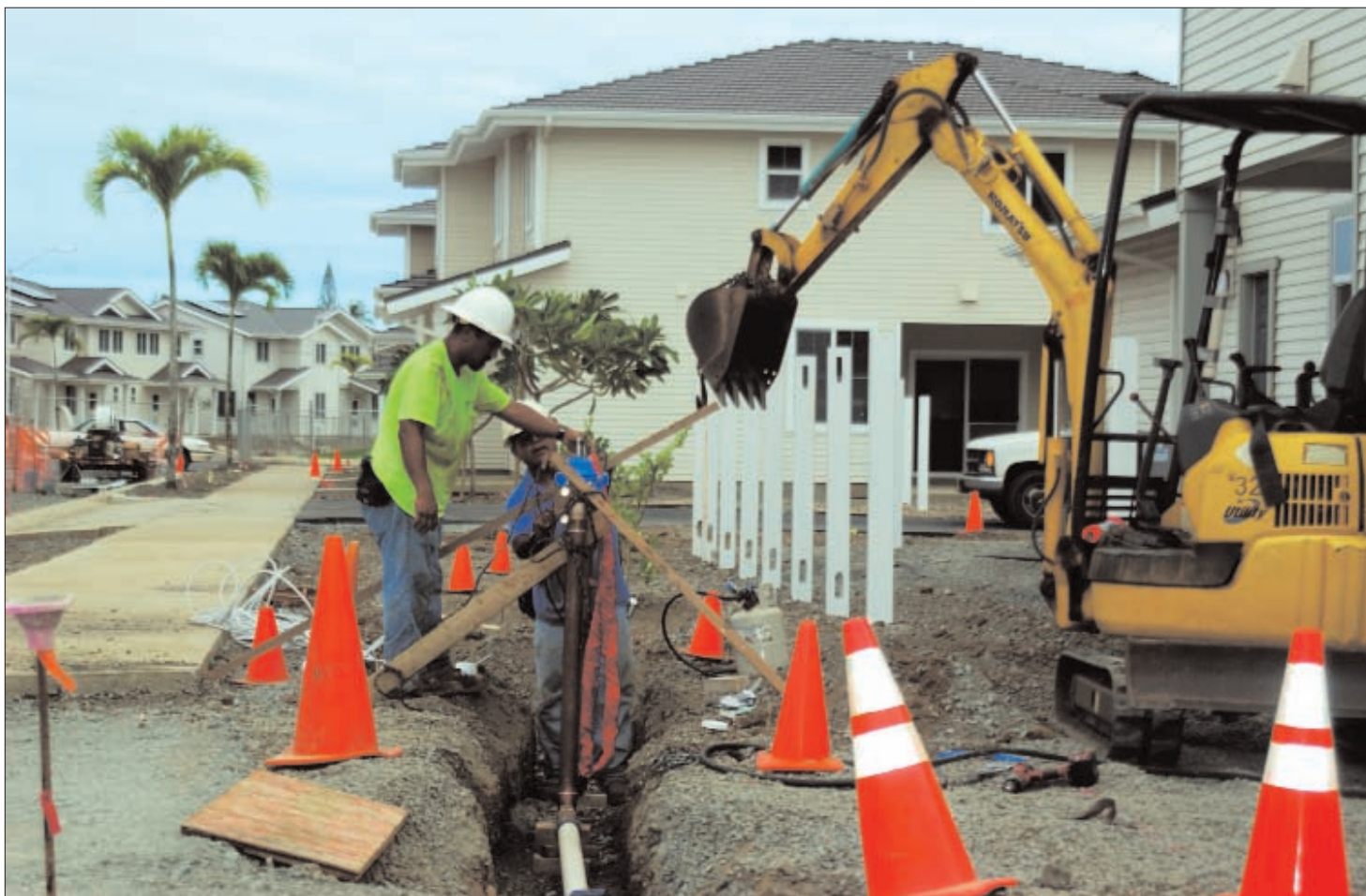
Construction workers install water pipes Wednesday for sprinkling systems near new homes in Waikulu neighborhood aboard Marine Corps Base Hawaii. A total of 190 units in Waikulu will be replaced with upgraded homes with the help of Forest City Military Communities Hawaii. Other renovated areas include the Mololani area, with more than 690 older houses rebuilt.
