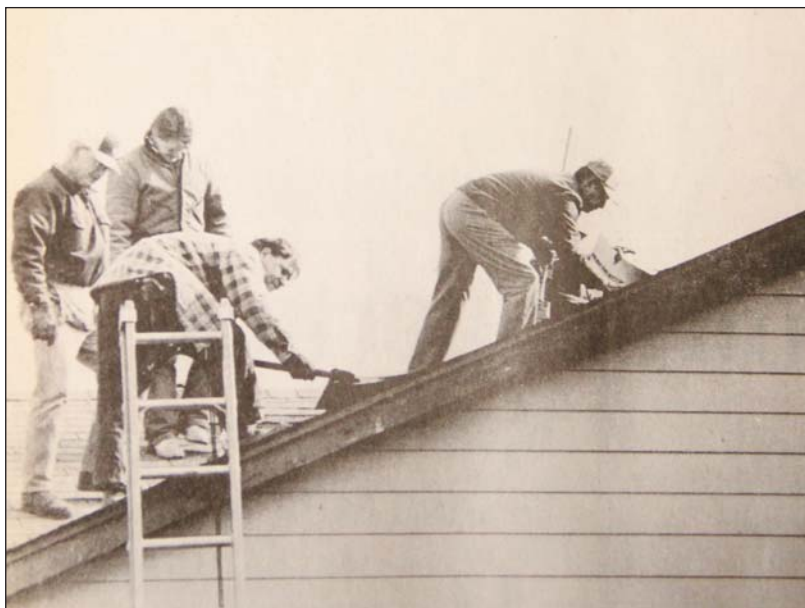
Above: Workers from the Directorate of Engineering and Logistics Operations replace shingles on a roof after a wind storm. Pictured from left are Charles Adams, William Blake, Clyde Sinclair and Malcolm Arnold.
