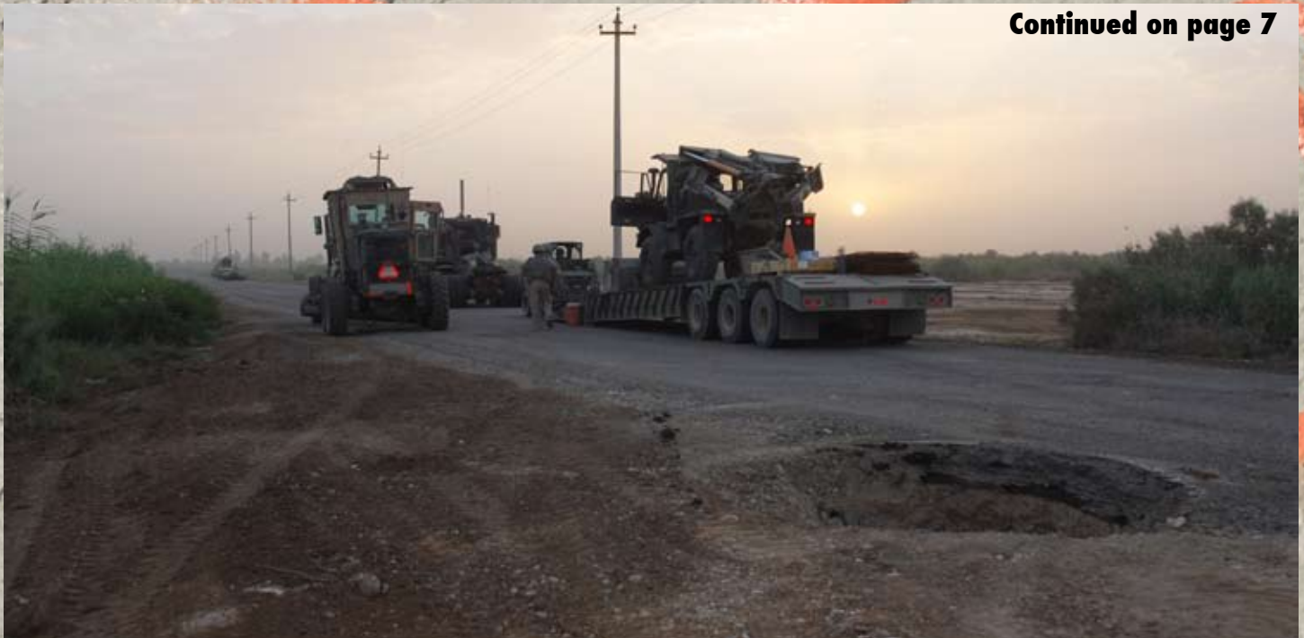
Members of 4th Platoon, Charlie Company, 875th Engineer Battalion begin to unload equipment to begin filling a large blast hole on Route Heather near LSA Anaconda. Rapid Crater Repair is a critical part of the battalion’s assured mobility mission in central Iraq.
