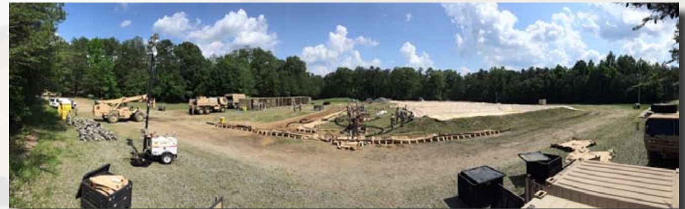
Approximately 140 soldiers from the 941st QM Co. U.S. Army Reserve -Puerto Rico are currently conducting their 2015 Annual Training at AP Hill, VA. As part of the exercise, the troops installed a FSSP operations (fuel system supply point) with about 75,000 gallons of fuel. (Photos provided by 941st QM Co. UPAR/ Release)
