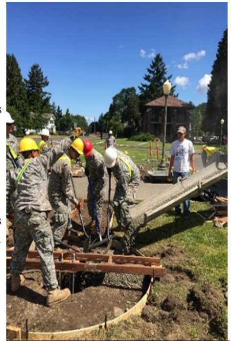
2nd Platoon placing concrete for the 7th Infantry Division Headquarters' BLDG flagpoles.
