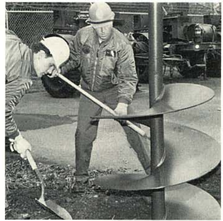
A1C Al Talley and TSgt. Jim Cornell "bust rocks" to keep their auger bit drilling freely. (Photo by MSgt. Harvey Tattel)
