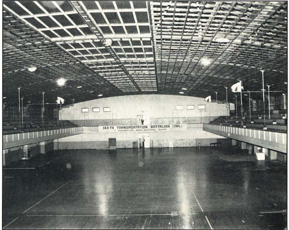
The work on the skylight is part of the renovation of the Tacoma National Guard Armory that sent the 144th Transportation Battalion looking for a temporary new home.
