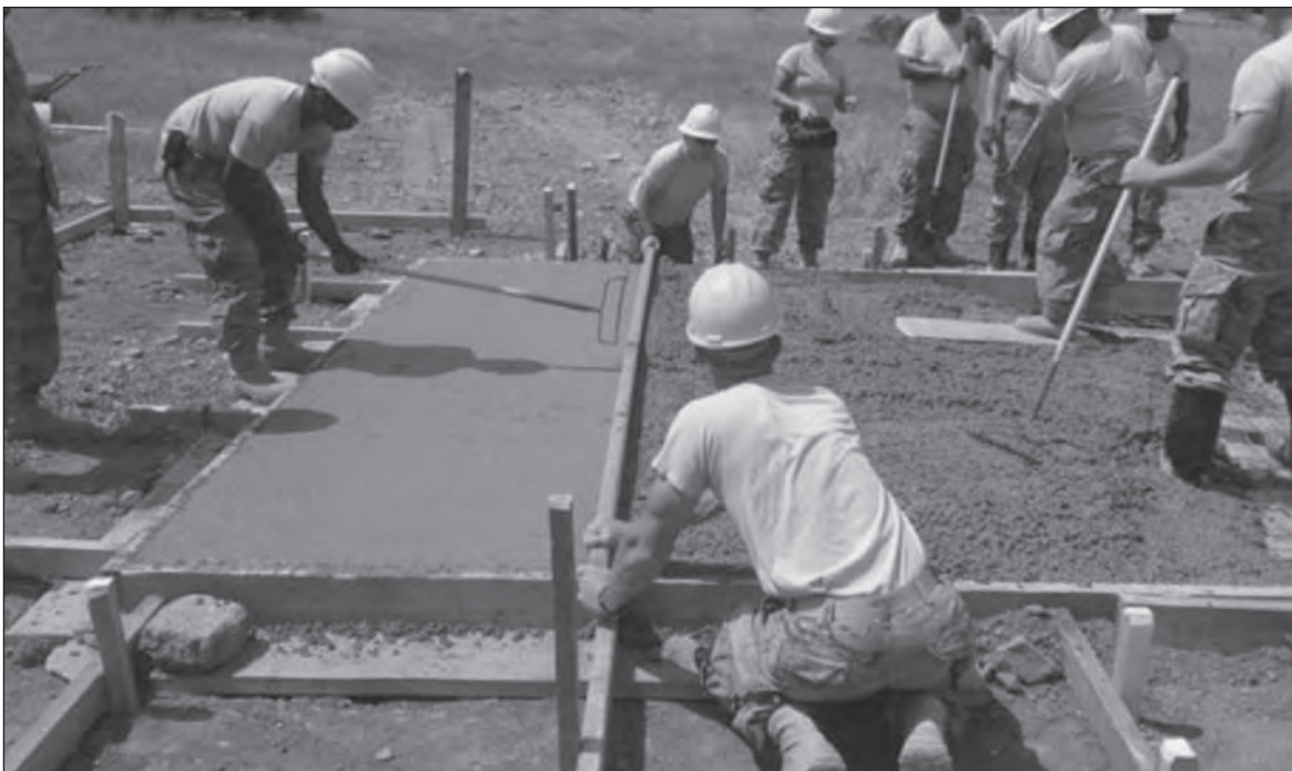
Soldiers from the 194th Engineer Brigade construct pads for a range storage building at the Novo Selo Training Area, Bulgaria.
