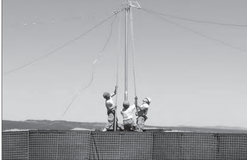
Soldiers from the Tennessee Army National Guard install part of a lighting protection system at the Novo Selo Training Area, Bulgaria.
