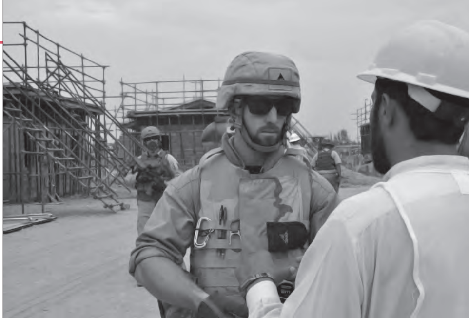
An American civil engineer meets with an Afghan engineer at a building site to make sure that construction is progressing according to the International Building Code and the plans and specifications for the site.
