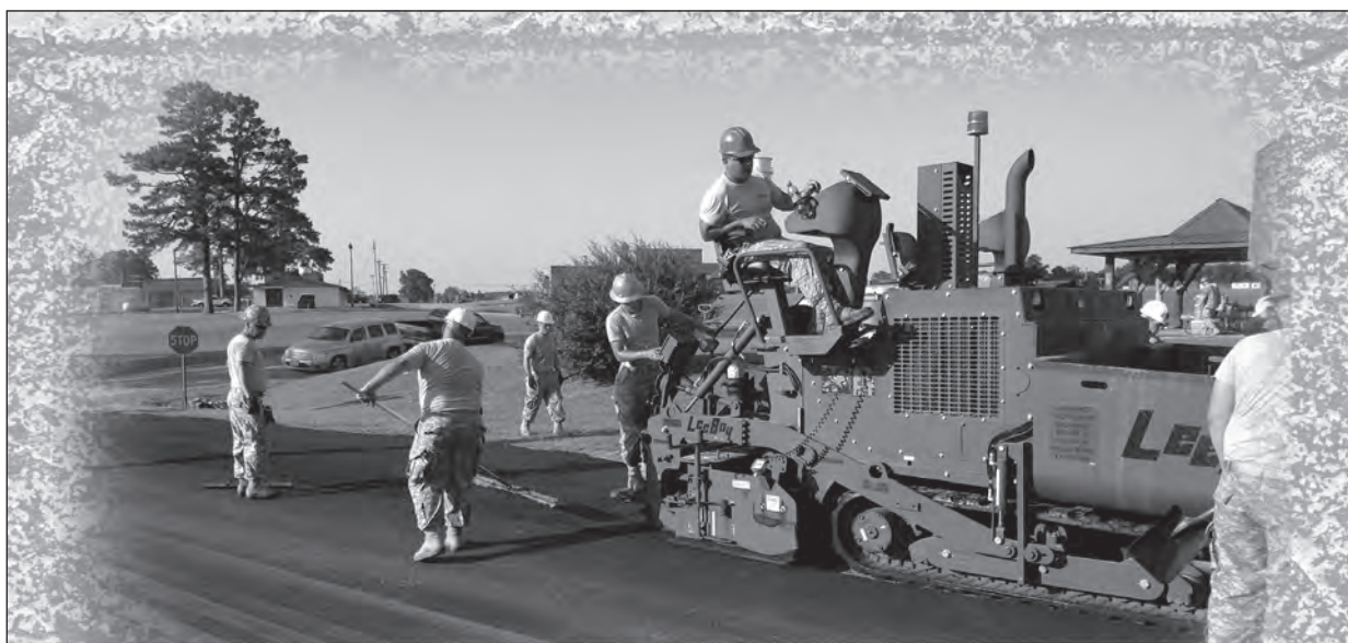
Soldiers from the 255th Engineer Detachment (Asphalt), a unit of the 230th Engineer Battalion, Tennessee Army National Guard, conduct paving operations at the Milan Volunteer Training Site, Lavinia, Tennessee. The Soldiers were some of the 36 detachment members who took part in the annual training. They paved two parking lots and three driveways, using 805 tons of asphalt in the process. The site, midway between Memphis and Nashville, is used by all Tennessee Army National Guard units; Regular Army units from Fort Campbell, Kentucky; U.S. Navy and U.S. Air Force Reserve Officer Training Corps cadets; sheriff departments from across the state; and local police departments and special weapons and tactics teams.
