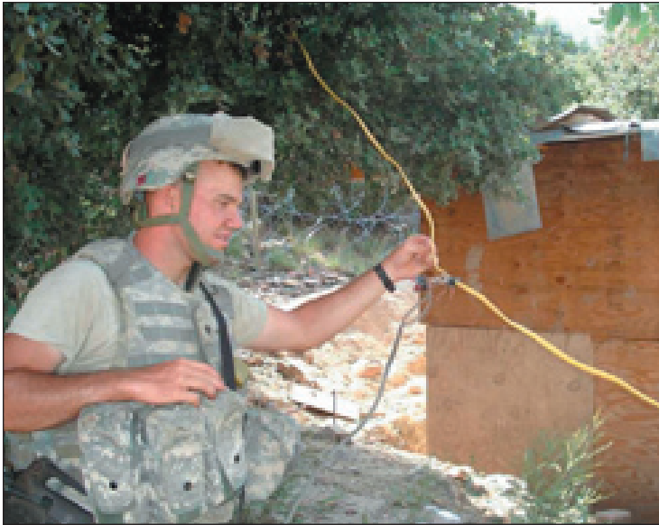
Spc. George Hart, 76th Engineer Company, performs electrical wiring inspections during winterization projects on an outpost. Courtesy photo
