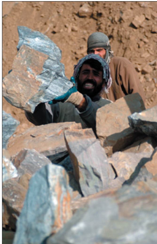
An Afghan construction worker piles rocks on the back of a truck for use in the building of Salang’s newest district center. The Bagram PRT visited the construction site to assess the progress of the project.
