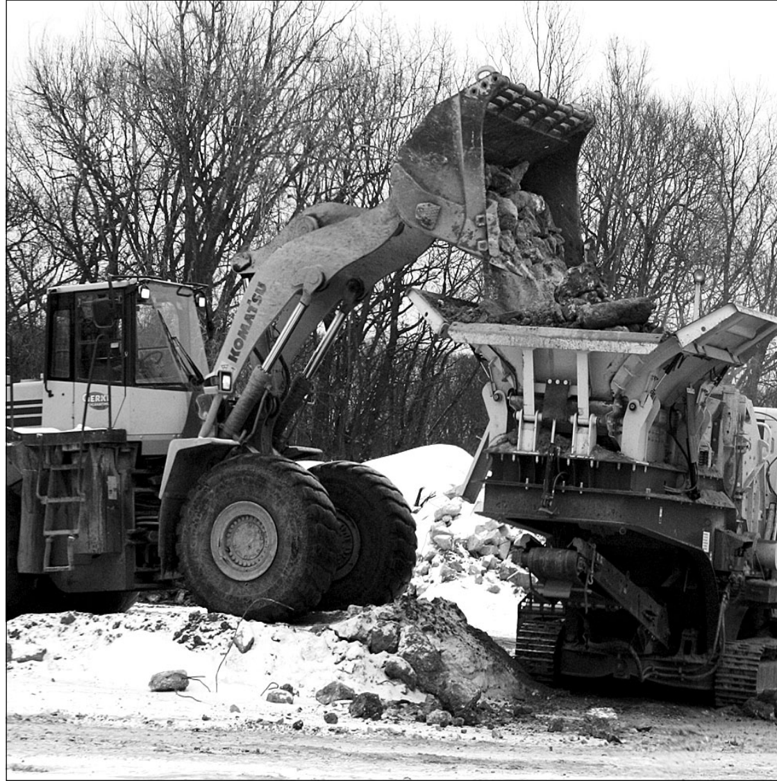
A contractor uses a loader to fill a rock crusher at an area on Fort McCoy's North Post.
