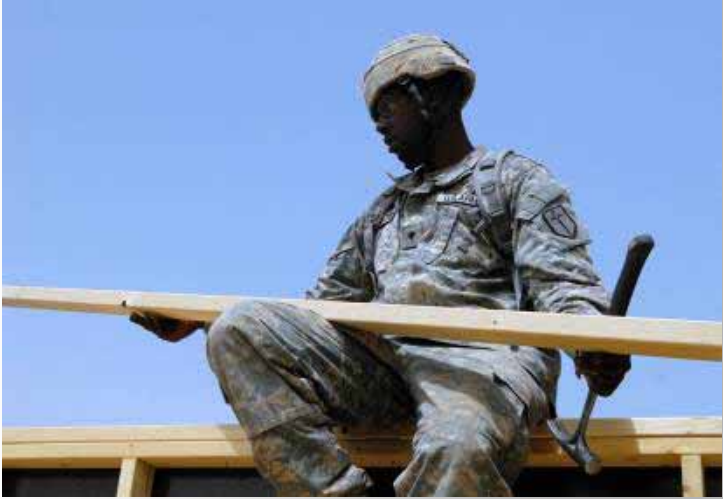
Highland Park, Mich. native, Spc. Issiah White prepares to install a double top plate to lock in the walls of his B-Hut at Combat Outpost Carver, located in the southeastern outskirts of Baghdad May 4.
