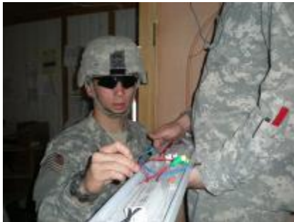
Spc. Alex Hunt of Juneau, Alaska prepares a light for installation. Hunt is an electrician.
