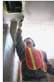
Miguel Ramirez, a drywall specialist with Precision Walls Inc., puts the finishing touches on a ceiling inside Cherry Point's Marine Dome, Feb. 17.
