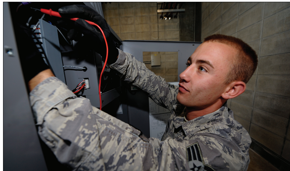
In this wire photo, Senior Airman Derek Hunter at Kadena Air Base, Japan checks circuits on an electrical system to promote efficiency. (U.S. Air Force photo/Staff Sgt. Jonathan Steffen)
